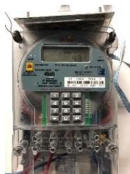
Figure 4. Digital kWh Meter
